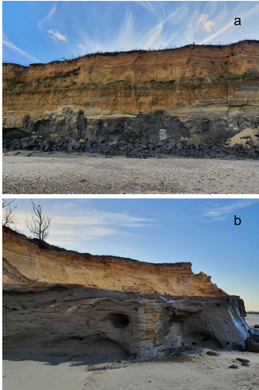
Figure 2.9 Soft substrate cliffs at Happisburgh (Figure a and b). Cliff vulnerability to erosion at Happisburgh is also exacerbated by surface runoff (observable in Figure b) (Photos: I Cotton).
