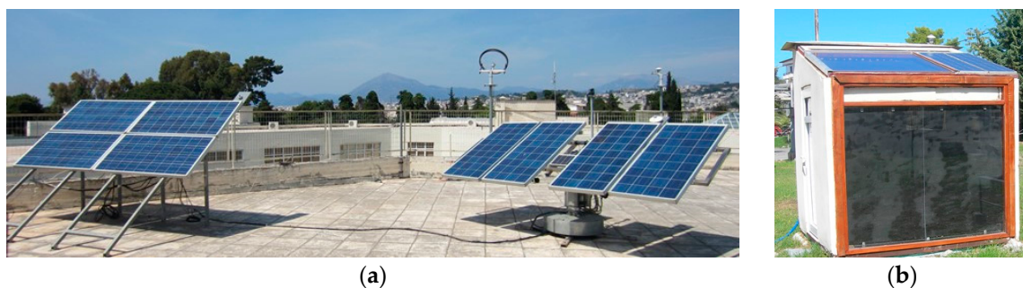
Figure 1. Experimental photovoltaic (PV) systems: (a) fixed-angle and two-axis sun-tracking PV; (b) building integrated photovoltaic (BIPV) test cell.
