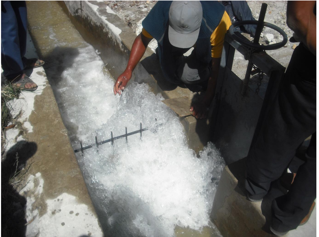
Figure 8.2 Photograph of lodged sluice-gates. Source: own.
