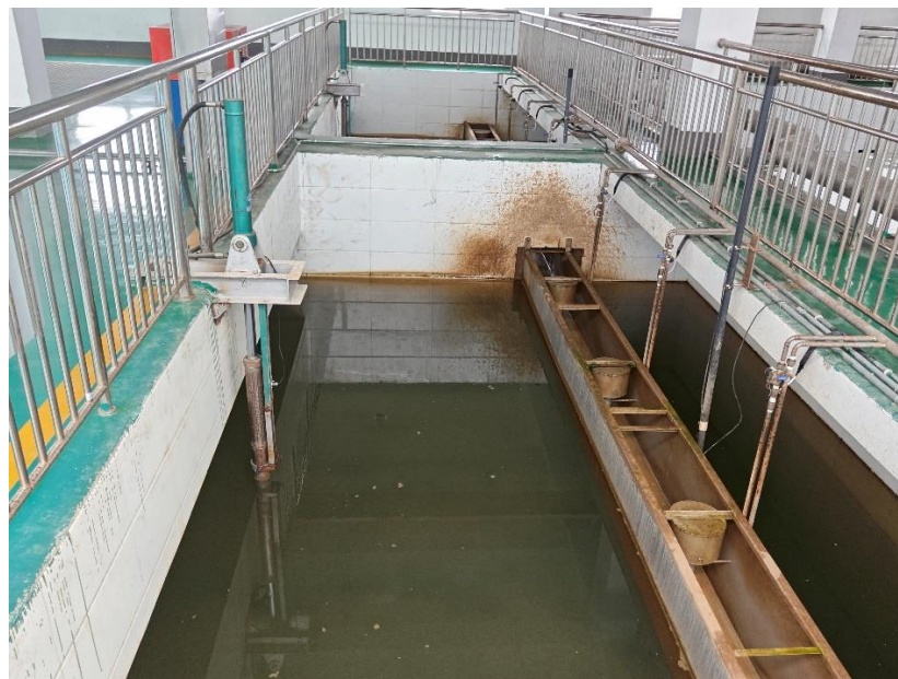
(b) The water purification plant.
