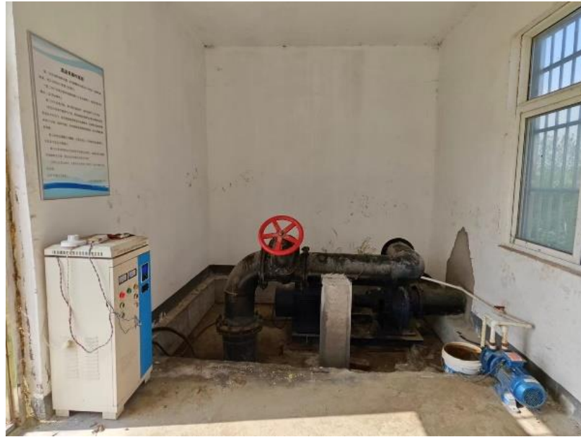
Figure 5.8. The pumping station built for the large family farm.
