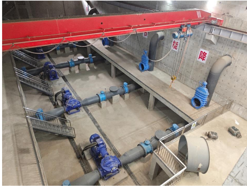
(a) The water intake pumping station.
