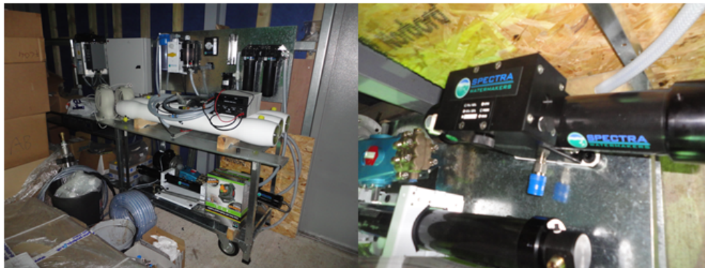
Figure 2.7.2: Preparing the system for international shipping. Note three RO pressure vessels, the full Spectra Watermaker kit including the Clark, a low pressure CAT pump, power converter and high-pressure pump controller.
