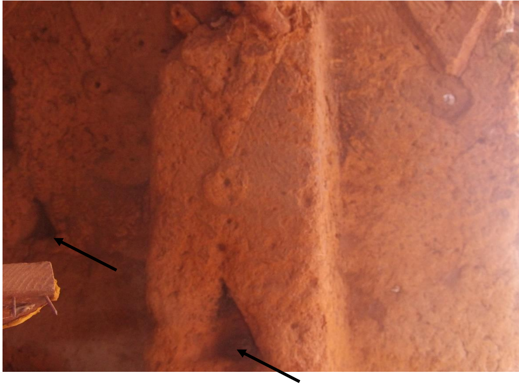
Figure 4.9. Mud wall showing cavity (indicated by black arrows) in a present-day house in Ilorin.
