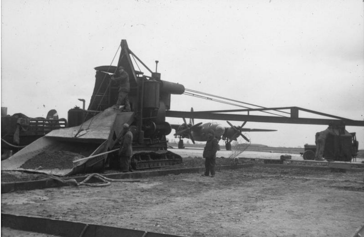
Fig.36 American construction engineers concreting runways. The image conveys the size and scale of specialised equipment used. 52
