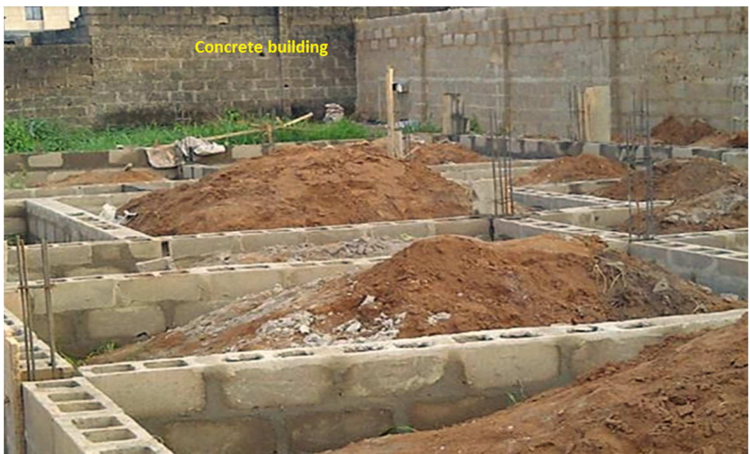
Figure 3.11: Additional form of building and materials used in the society (mud and concrete bricks).
