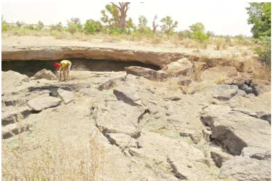
Figure 3.22: Collapsed clay mines in Garande and Faggo settlements.
