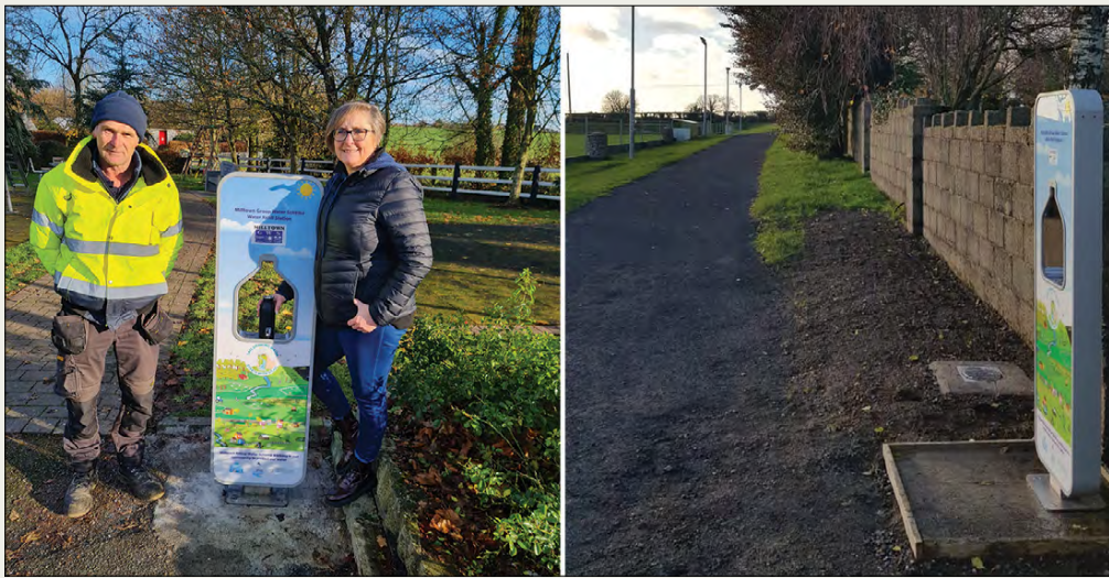
Examples of drinking water refill stations installed in Milltown Community GWS and Ballacolla GWS last year.
