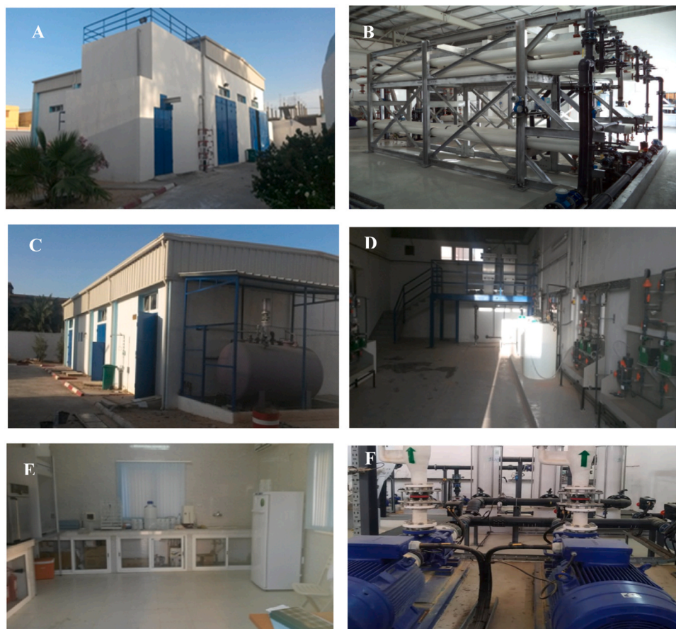
Fig. 2. Photographs of reverse osmosis desalination facilities in Ouargla province showing (a) exterior building, (b) membrane modules, (c-d) Chlorination building, (e) Analysis laboratory and (f) Pumping System.
